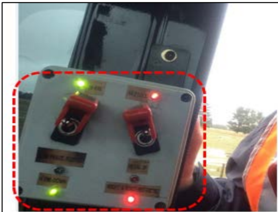
Figure 1. Two vertically-oriented toggle switches; 6 status lamps (of which 4 are shown illuminated); dymo-tape labels.
