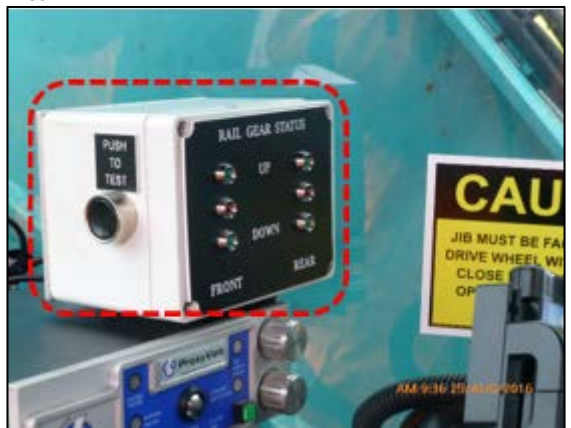
Figure 8. RGS status display only (controls located separately); 6 status indicator lamps; dedicated labelling; lamp test button function.
