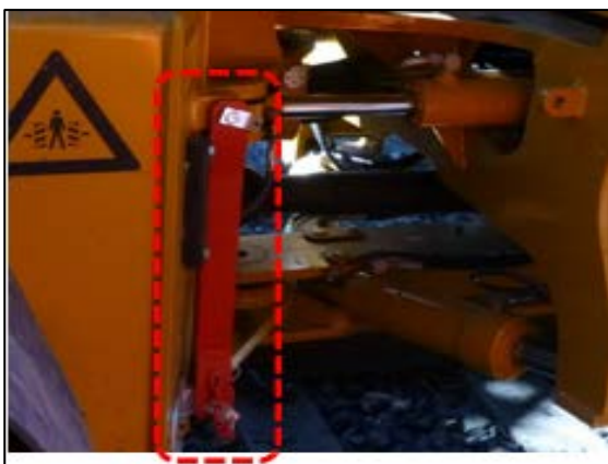
Figure 30. View clearly showing the pivot lock (red bar) not locked in place. The RRV was on the rails at the time. Notably, the pivot lock bar appeared new and showed no indication of use.
