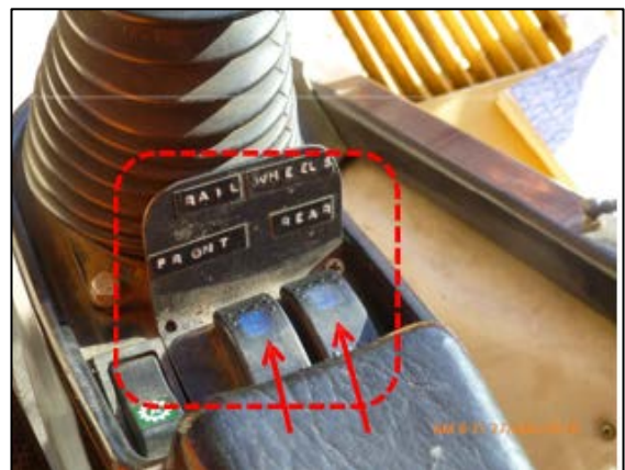
Figure 4. Two press switches (arrowed); switches appeared to contain blue-coloured embedded indicator lamps but these did not illuminate; dymo-tape labels.
